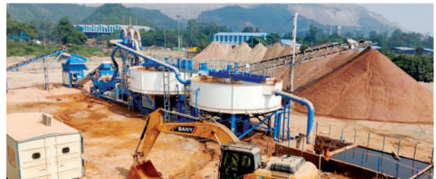
Sand Making Plant at Amlohri project of NCL.
