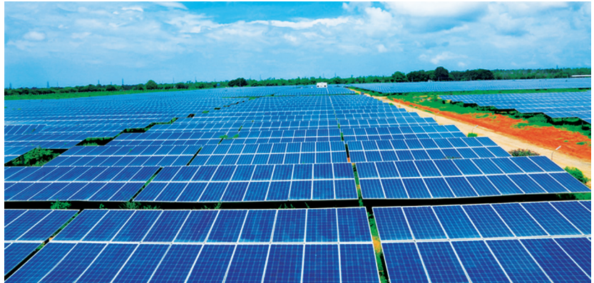
Solar Photovoltaic Power Project.
