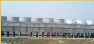
SUPER THERMAL POWER PROJECT AT NAGPUR, MAHARASHTRA
