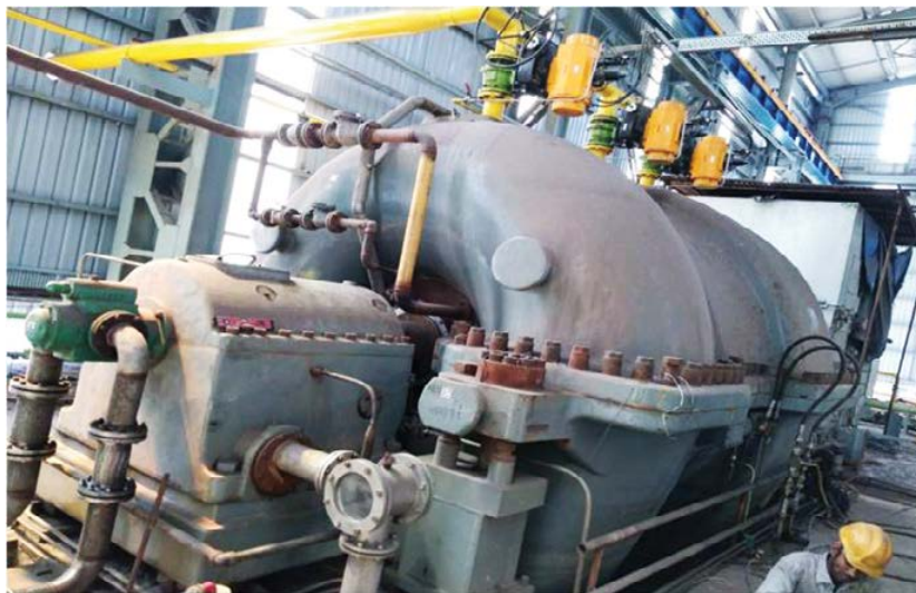
Top Recovery Turbine #BF 8, Bhilai
