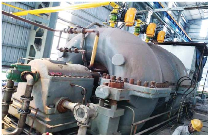
Top Recovery Turbine #BF 8, Bhilai
